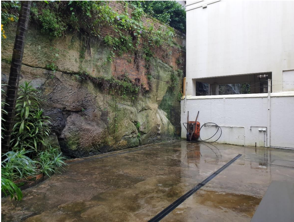
Figure 4: Rear yard of the subject site, including sandstone rock cliff face and masonry retaining wall, looking north-west
